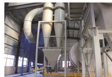
除尘行业 Dust removal industry
